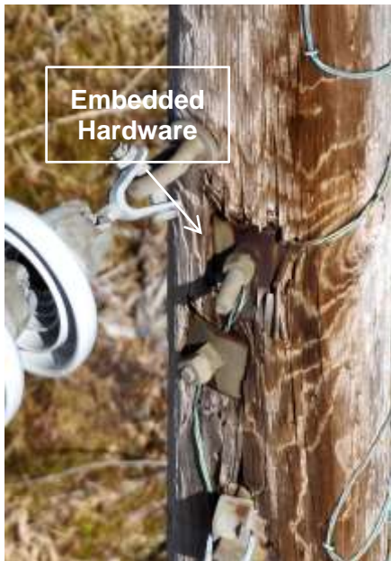
Figure 3 Hardware embedded in rotting pole
