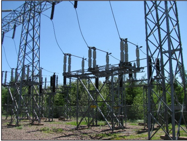
Figure 7: Lattice Structure Substation
