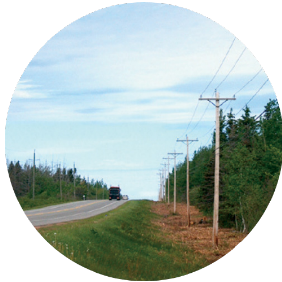
Vegetation and trees have been cleared from power lines to ensure correct distance and safety requirements are in place.
