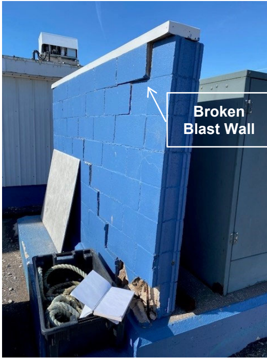
Figure 1 Padmount transformer broken blast wall
