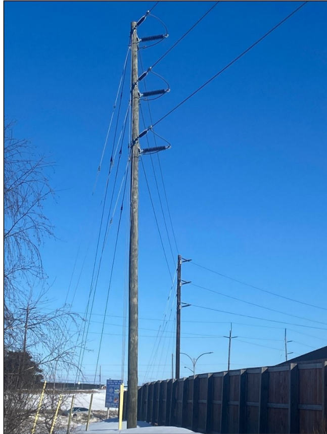
Figure 5: Double-Dead-End Light-Angle Structure
