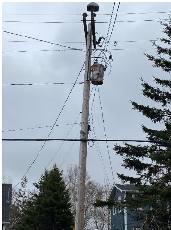
Figure 7 Inadequate neutral spacing for upgrading transformers
