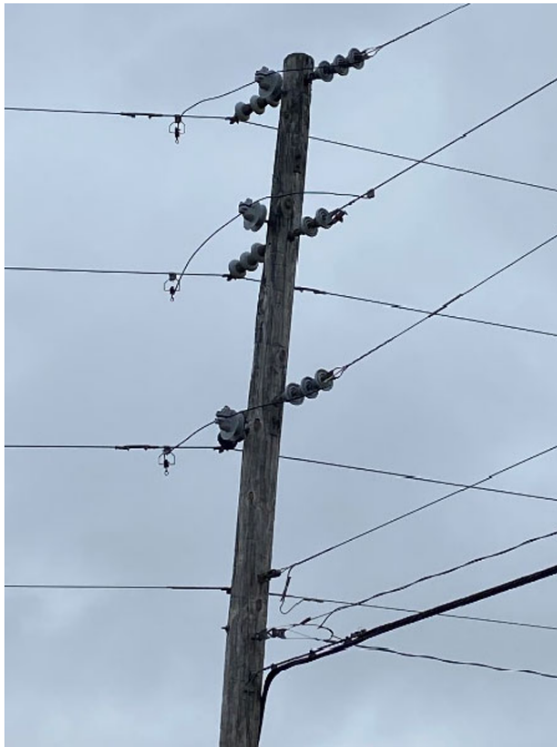
Figure 5 Deteriorated pole with porcelain bell insulators
