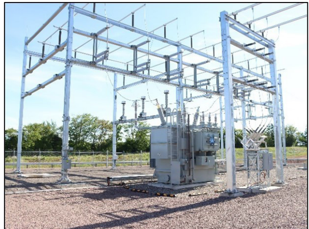
Figure 10: Structural Steel Substation
