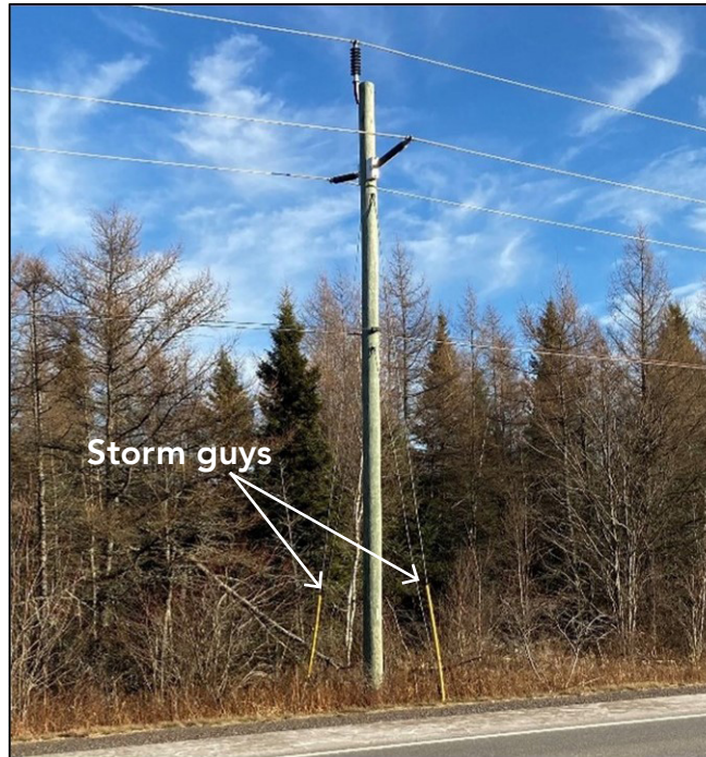
Figure 4: Two-Way Storm Guys on Transmission Structure
