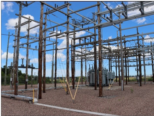
Figure 9: Wood and Fibreglass Substation
