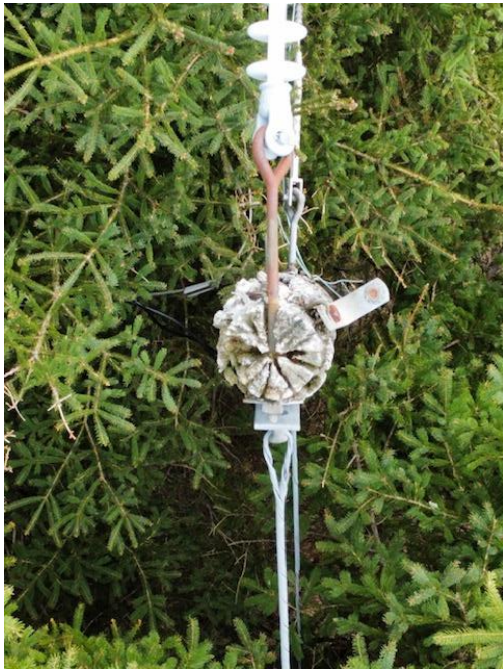
Deteriorated pole top with primary hardware exposed.
