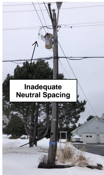
Figure 3 Inadequate neutral spacing and rusted transformer.
