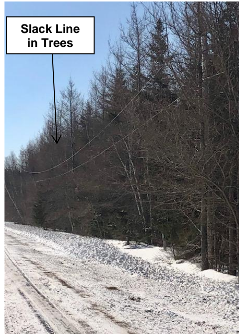
Primary line slack and laying in trees.
