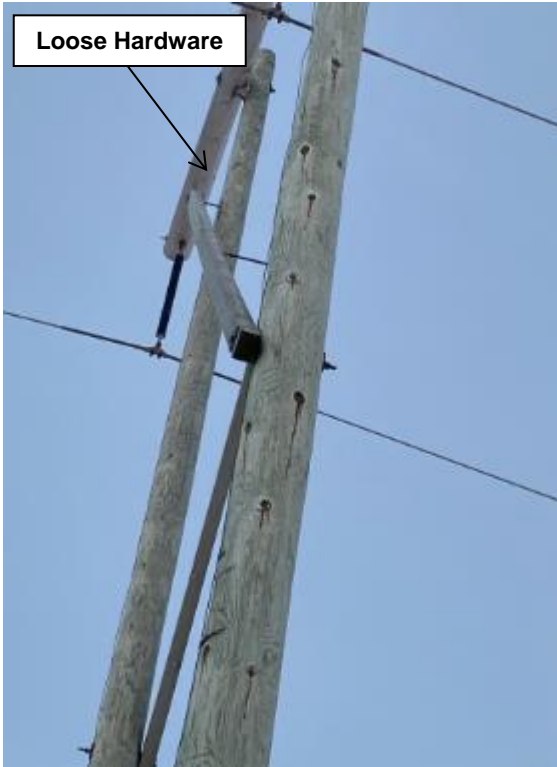
X-brace detaching from pole.
