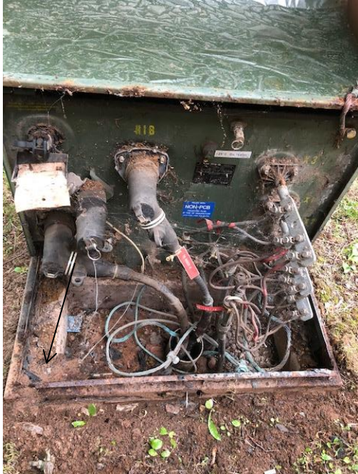
Rusted padmount transformer with sunken concrete pad.
