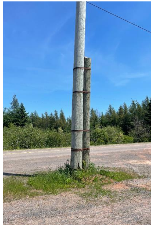
Cracked, damaged pole.
