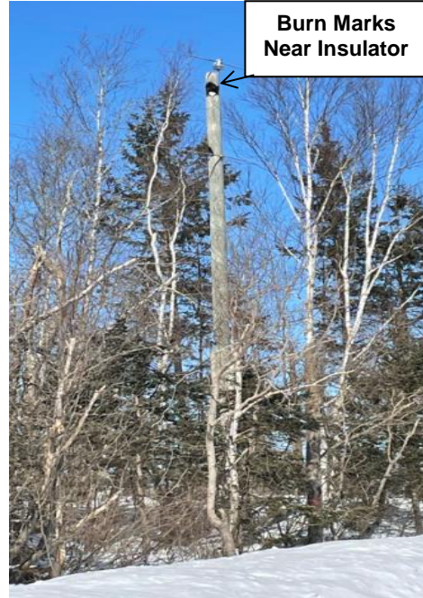
Burn marks from a failed insulator.
