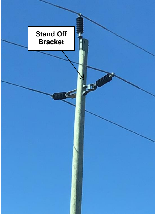
Stand-off brackets on insulator to be replaced.
