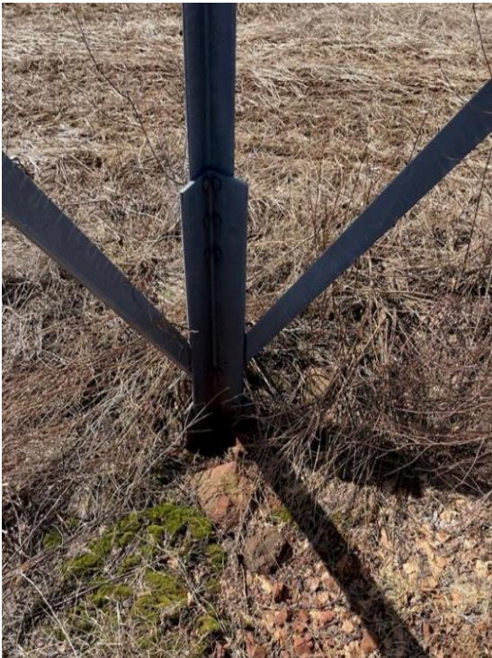
Sunken tower base.
