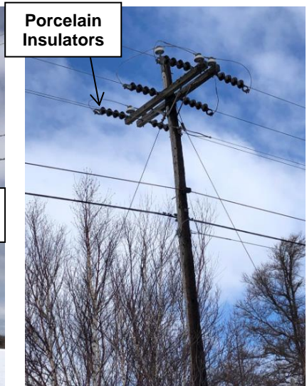
Figure 4 Aged porcelain bell insulators.
