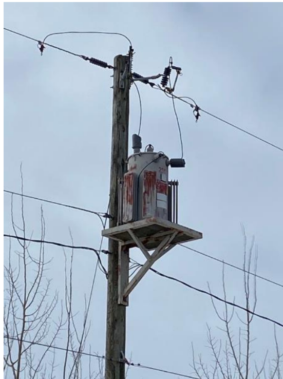
Figure 2 Aged pre-1982 step-down transformer.
