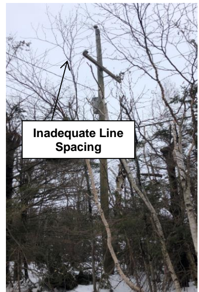
Figure 4 Structures with inadequate line spacing that do not meet current standards.
