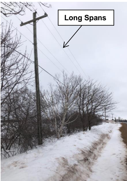
Figure 2 Long spans that do not meet current standards.
