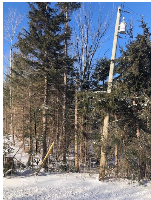
Slack anchor allowing the pole to lean.
