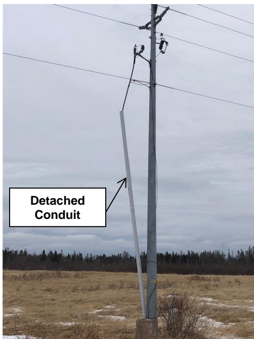
Underground primary conduit unattached from pole.
