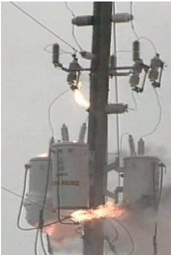
Example of a pole fire
