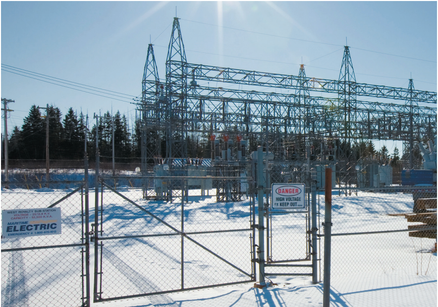
Maritime Electric Substation
